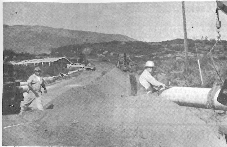
WATER PIPELINE GOING IN AT E. VICTORIA & HWY 80, IS TODAY COVERED. NEW BAPTIST CHURCH AT LEFT. VIEJAS MOUNTAIN IN BACKGROUND.
