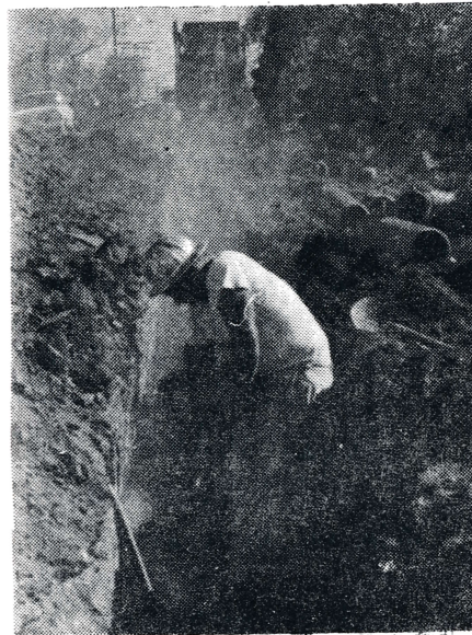
RUDY FLORES OF EC DRILLING INTO HARD BLUE GRANITE FOR A BLAST IN A SECTION OF PIPELINE DITCH ON ALPINE HEIGHTS ROAD. INSPECTOR K.W. OPPENHEIMER OF RIO SD MWD IS ON JOB SEEING THAT ALL GOES CORRECTLY.
